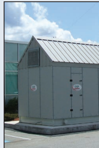
This Aircogen combined heat and power system has reduced the company's energy costs and greenhouse gas emissions.
