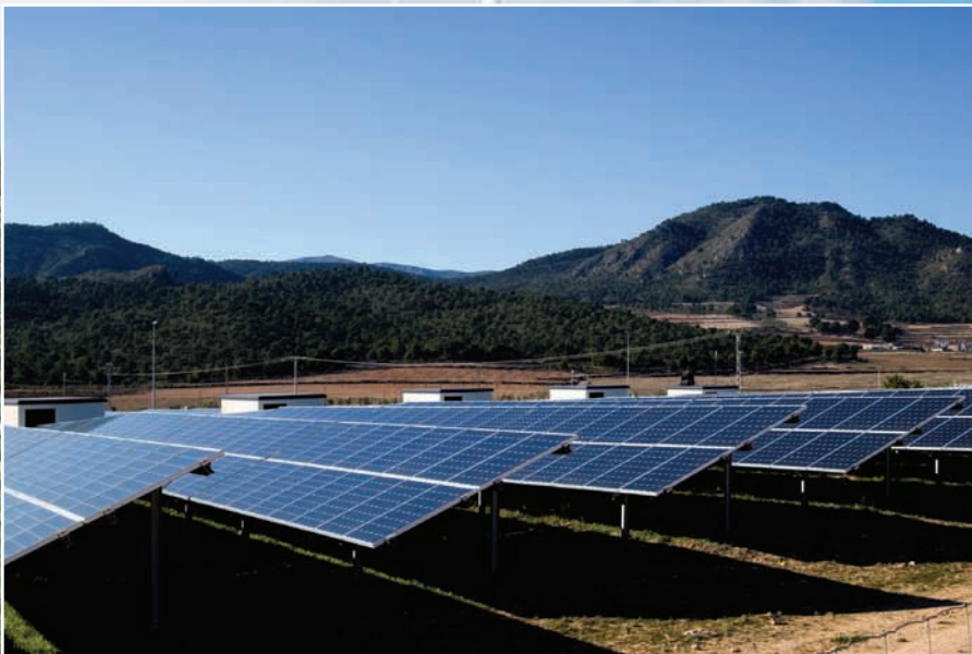
Solar power plant.
