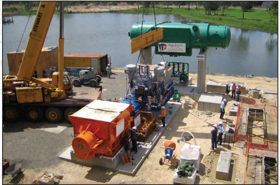
A 25.5 MW Peter Brotherhood steam turbine being installed at the Isis Central Sugar Mill in Childers, Queensland, Australia..
